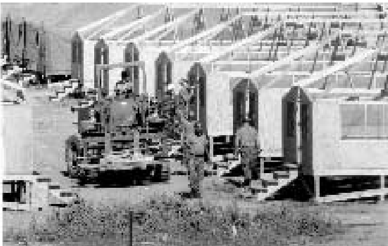
Navy SEABEES use contingency construction skills to construct strong back tent villages for Cuban migrants during Operation SEA SIGNAL.
